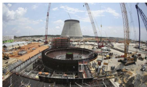
Georgia Power Nuclear Plant
